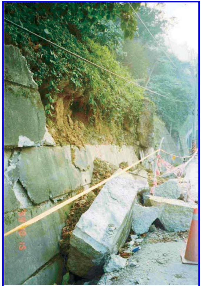
Fig. 4. Outward movement of the gravity wall along construction joint.
