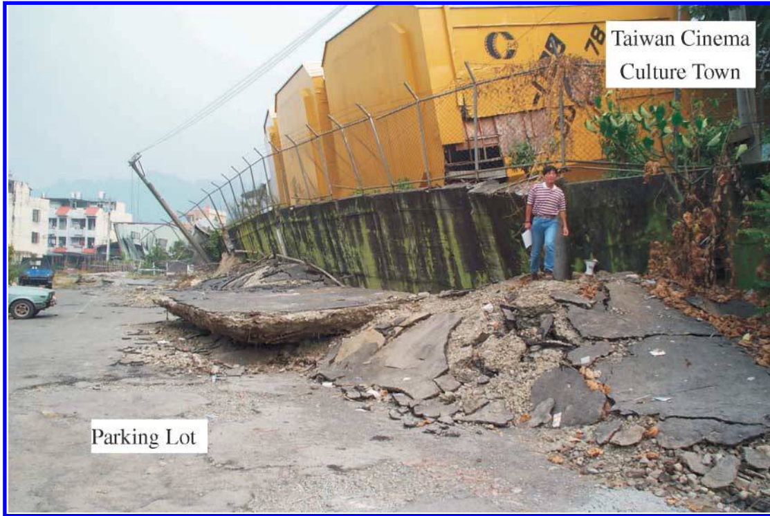
Fig. 14. Sliding and overturning of retaining wall at site 3.
