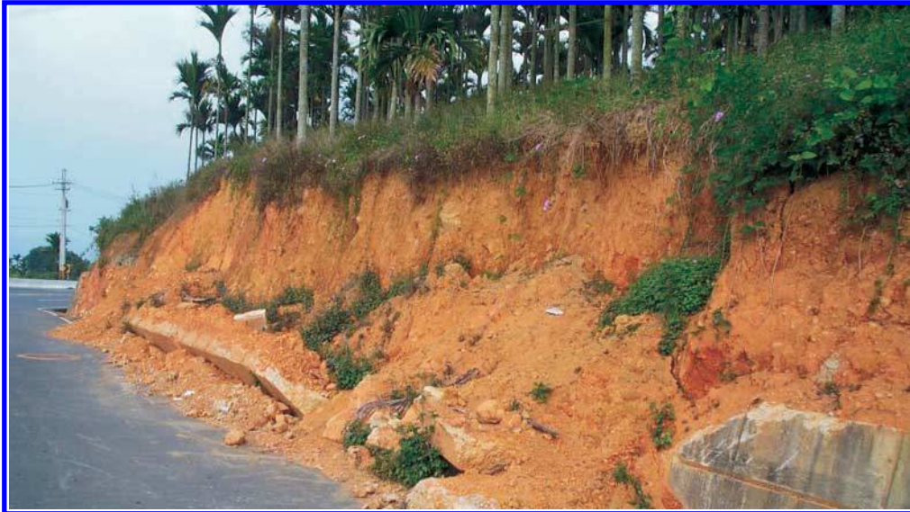
Fig. 9. Overturning of gravity wall at site 2.
