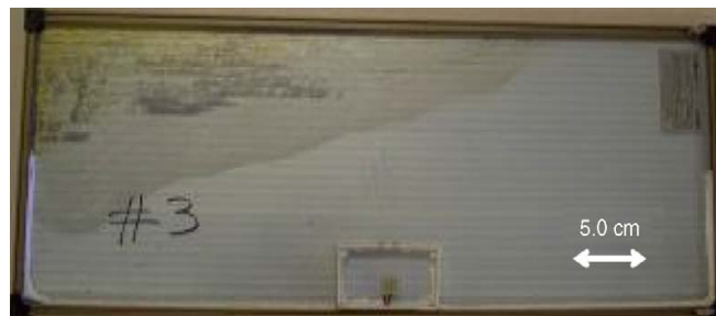
Fig. 2-5 Photograph of rear of module showing delamination and moisture ingress. [23]
