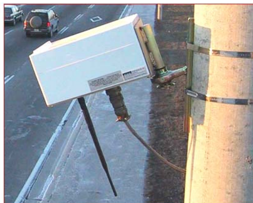
RTMS (Remote Traffic Microwave Sensor) radar
